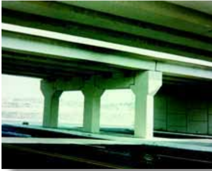
Piers and abutments can also be made of precast concrete pieces quickly assembled in the field.
