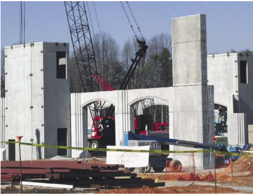
Fig. 10. Erection of the first precast concrete walls. (Courtesy of Don Brown, Metromont Corporation)
