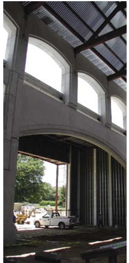
Fig. 12. An interior view showing the precast concrete arch in position. (Courtesy of Randy Davis, Design/Build Engineers, Inc.)
