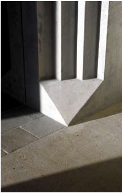
Fig. 18. Close-up view of foot of column in the narthex. Precast concrete is particularly effective as a foil to the slate and salt-finished concrete floor. (Courtesy of Brian Dressler)
