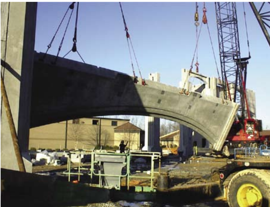
Fig. 11. Two cranes hoisting the 77,000 lb (35,000 kg) precast arched spandrels. Note the special rigging with numerous pick points. (Courtesy of Jeff Hargett, Metromont Corporation)
