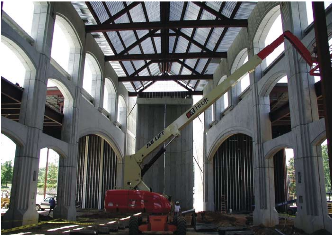
Fig. 7. Steel roof trusses bearing on precast concrete walls required careful attention to detail, as the precast concrete walls were not parallel. (Courtesy of Design/Build Engineers, Inc.)
